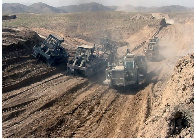
August 3, 2005 - Army engineers from AK-based Company C, 864th Engineer Combat Battalion, level a portion of the nearly completed 117-kilometer TK Road, stretching from Kandahar to Tarin Kowt, Afghanistan. The road will link vast, difficult-to-access portions of the country, fostering commerce and facilitating travel to election polling sites next month.. – Photo by 1 st Lt. Laura Walker.
